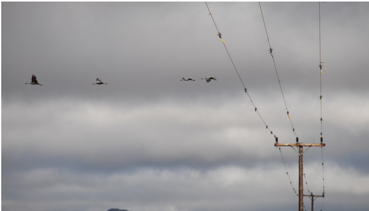
Blue Cranes passing over a Distribution line marked with bird flappers. Photo credit: Marianne Golding
