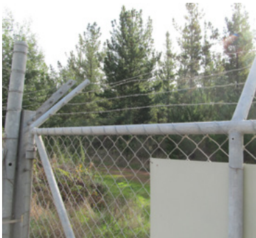
The section of the fence the baboons use to enter and exit the substation.
