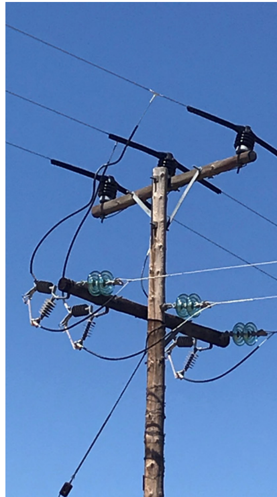
Raptor protectors and insulated jumpers on a distribution pole.
