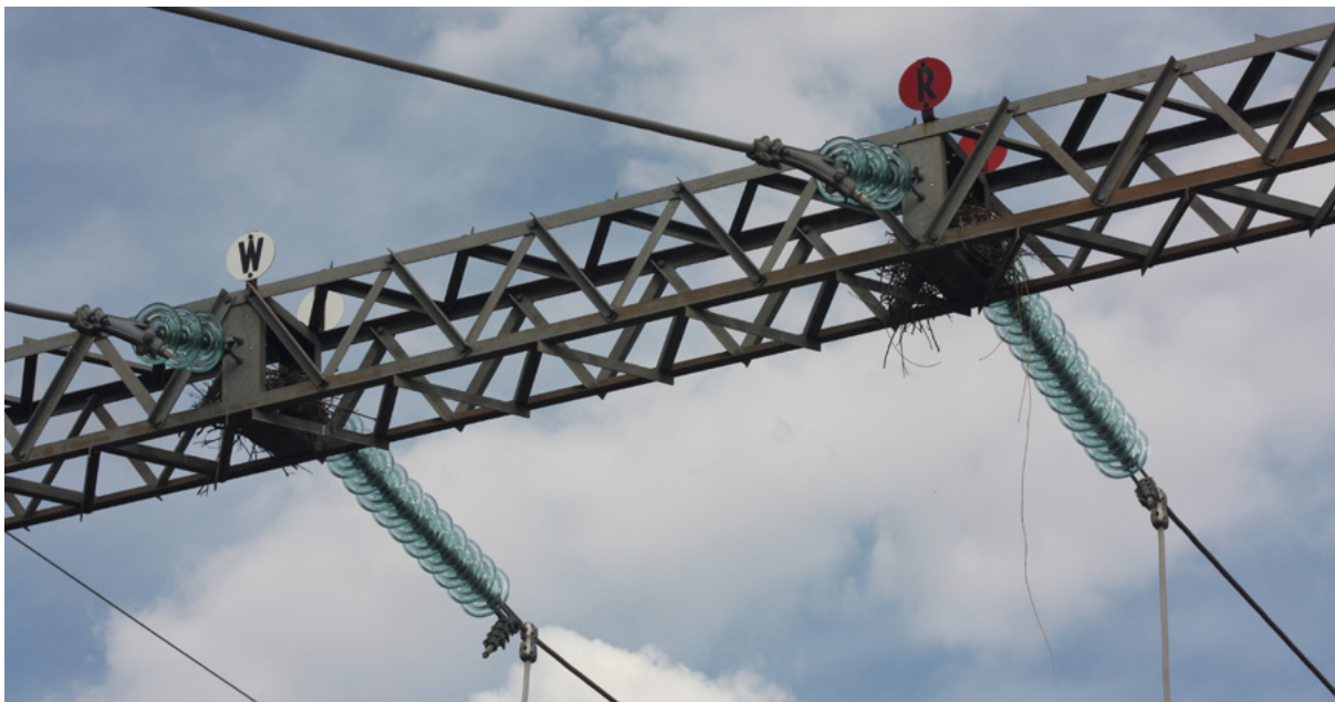
Bird nests are often found in substations as they provide a safe and secure location for breeding birds.
