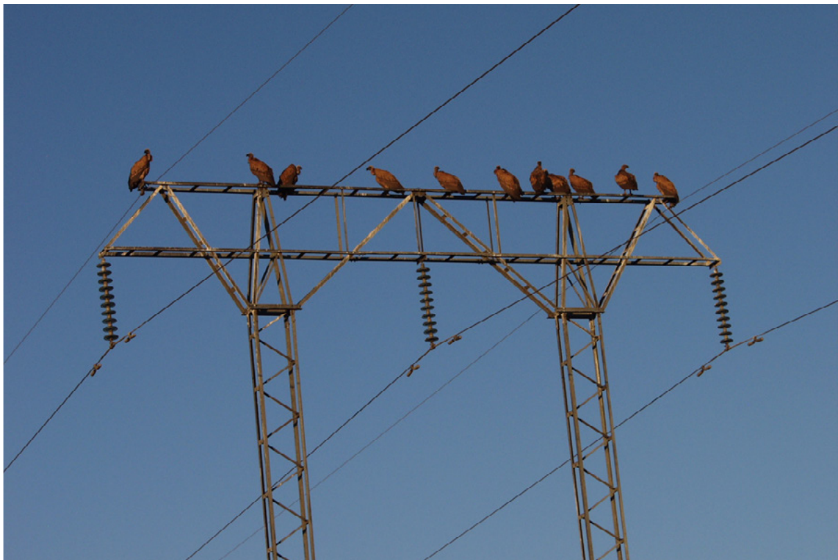
Birds perching on electrical structures results in a build-up of pollution on the structure and live components.
