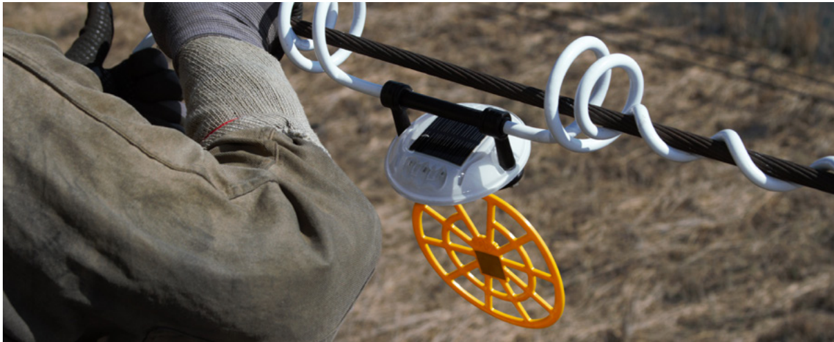
The OWL nocturnal bird flight diverter with flashing LED lights, intended to be visible to nocturnal flying birds so that they can avoid colliding with the power line. Photo credit: Matt Pretorius
