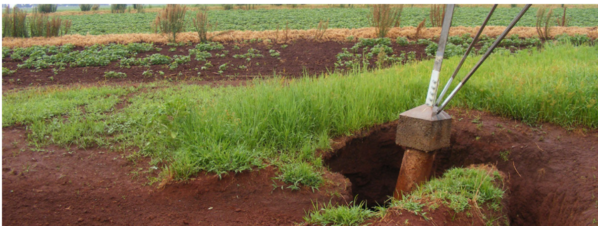
Porcupines digging holes next to the base of a Transmission line, compromising the integrity of the structure. Photo credit: Constant Hoogstad
