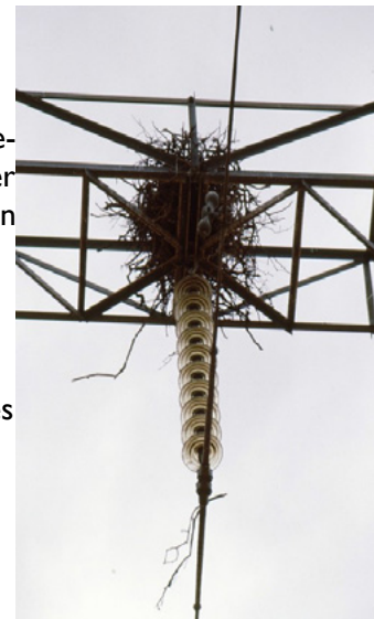
Crow's nest located above insulator on a transmission line. This nest has the potential to be problematic and cause outages. Photo credit: Constant Hoogstad
