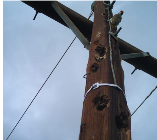
Woodpeckers often make multiple holes in poles, severely compromising their stability. Photo credit: the EWT
