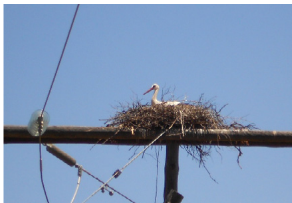
White Stork nesting on a distribution pole at the entrance to a substation. Photo credit: Eskom
