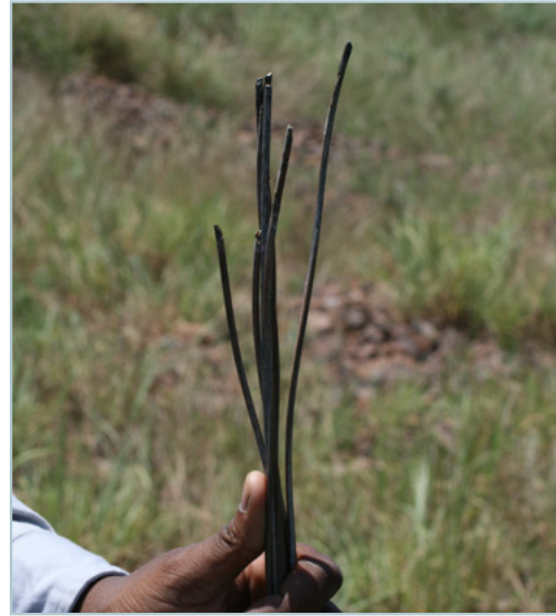
Figure 3: The earth/shield wire appears burnt. Vulture activity is unlikely to cause this type of damage.
