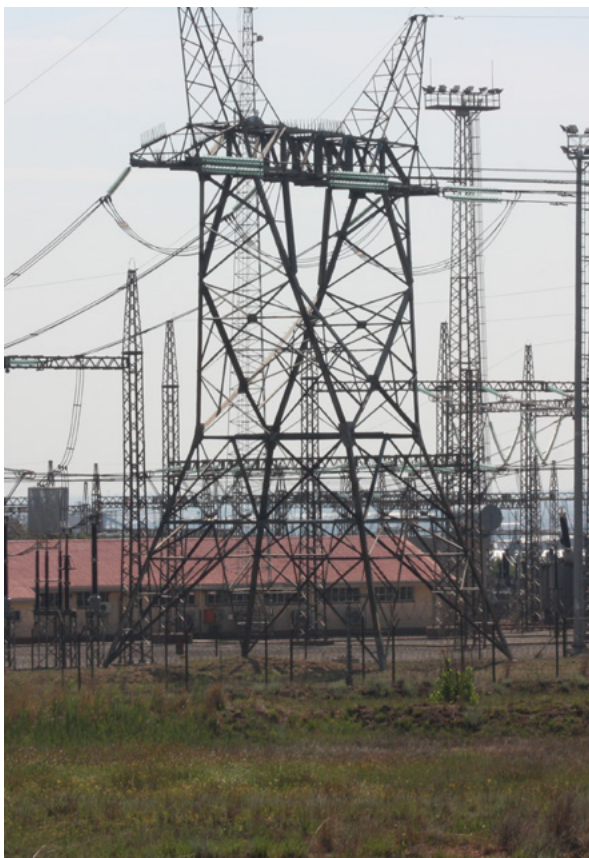
Typical substation in Africa which often provides a safe haven for wildlife. Photo Credit: Constant Hoogstad
