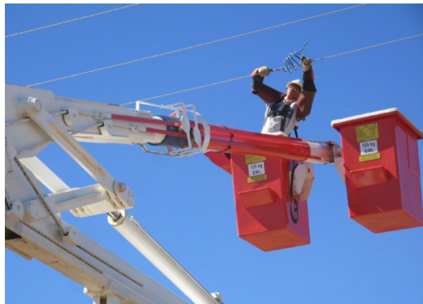
A live line team installing bird flight diverters on a distribution line. Photo credit: Megan Diamond
