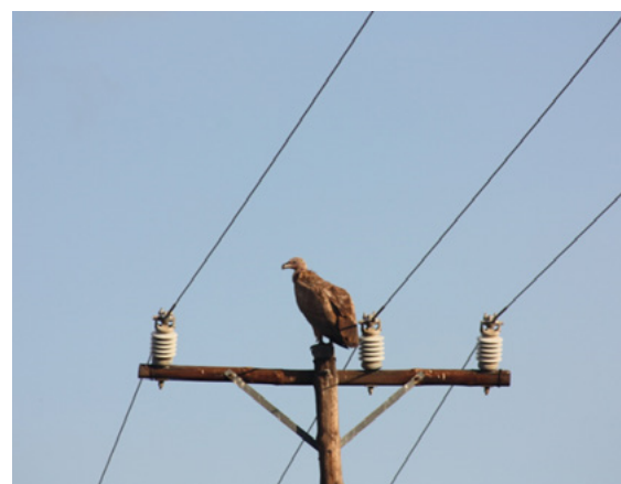
White-backed Vulture perching on an unsafe T-pole structure with a very high electrocution risk.
