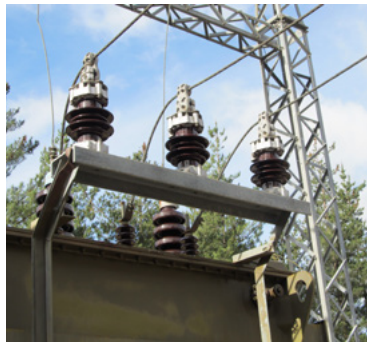
There is currently no insulation on the live components within the substation.
