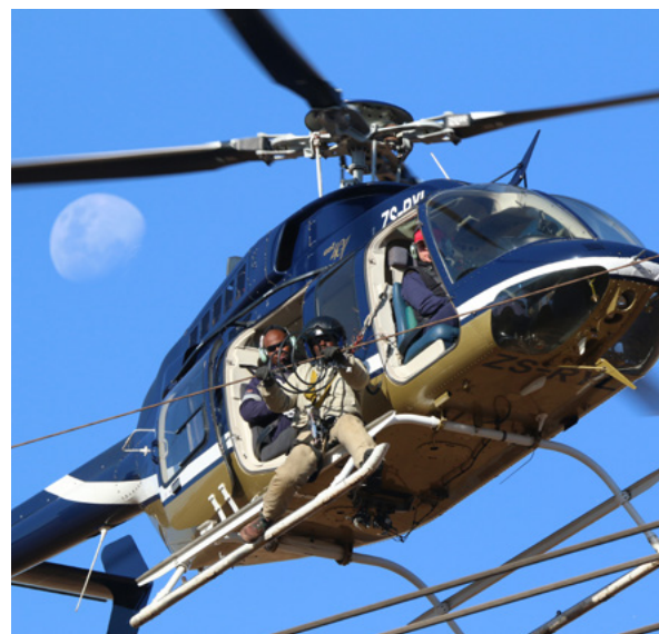
A utility crew retrofitting a power line with markers Photo credit: Constant Hoogstad
