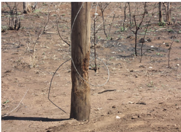
Wood distribution pole compromised due to rubbing by large mammals. Note the earth wire being ripped off the structure.
