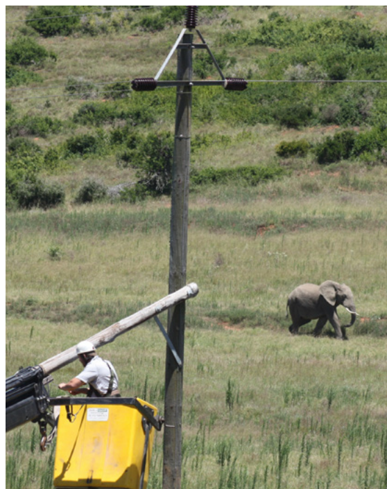
Maintenance on wood distribution poles in a National Park. Photo credit: Constant Hoogstad
