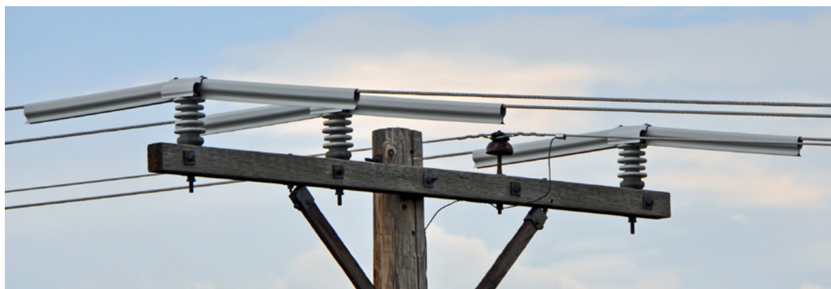
Raptor guards on a wooden distribution line in the USA. Photo credit: Lourens Leeuwner
