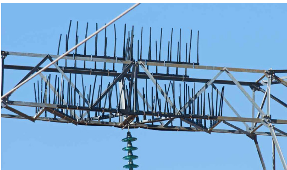
Bird guards placed above the center phase on a transmission tower to minimize streamer and pollution problems. Photo credit: Matt Pretorius
