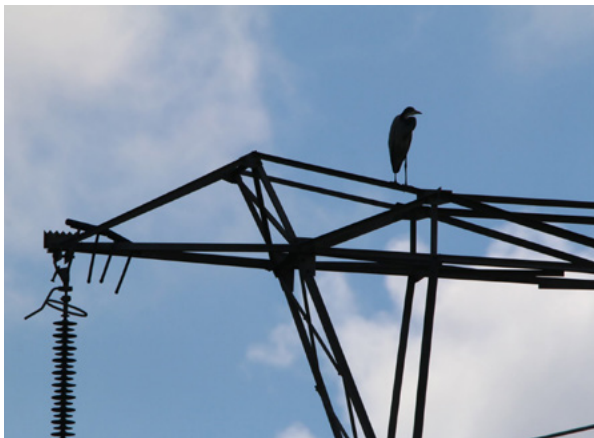
Example of bird guards installed using incorrect cable ties, causing the product to fail. Photo credit: Constant Hoogstad
