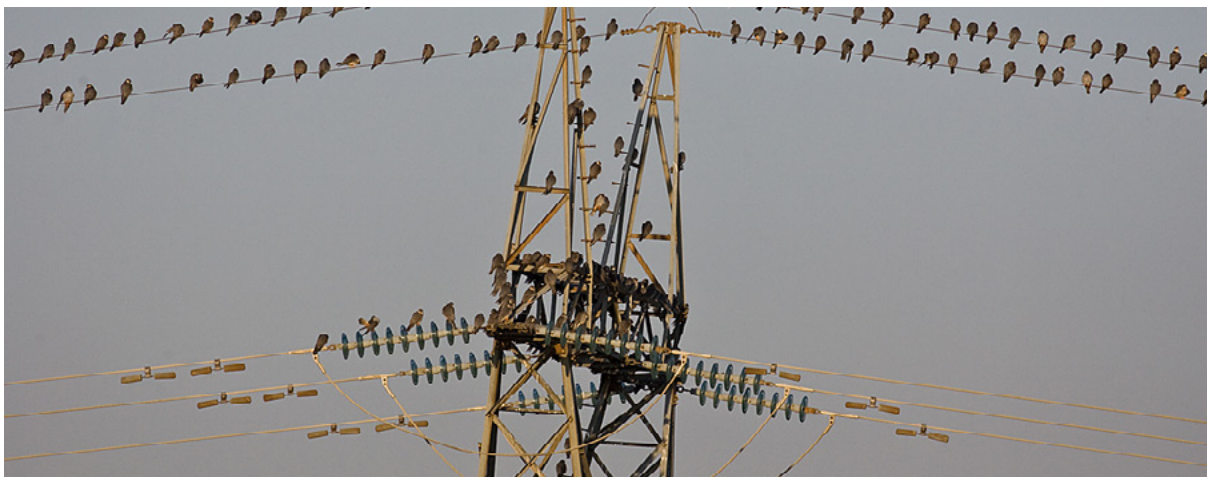
Amur Falcons roosting on a transmission structure. Photo credit: Andre Botha
