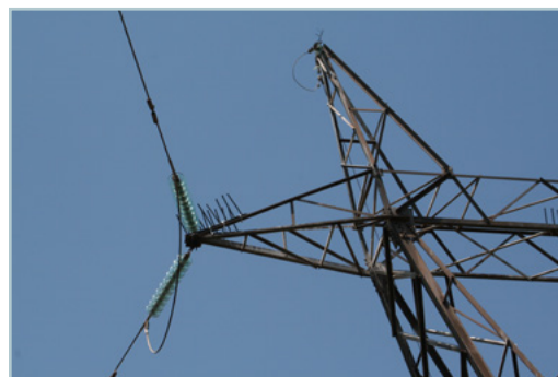
Figure 2: The insulator strings were not heavily polluted, suggesting that the bird guards were at least somewhat effective. Photo credit: the EWT
