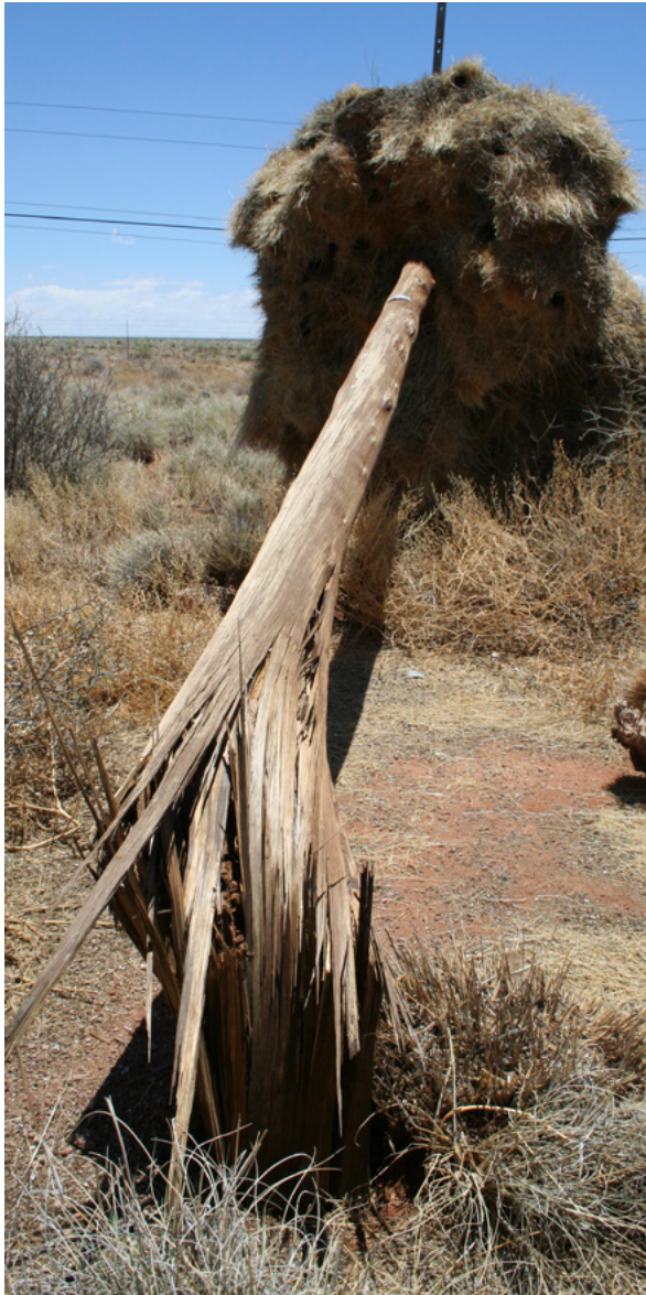
Sociable Weavers build nests that often weigh up to 1,000 kg, causing wood distribution poles to break due to the weight. Photo credit: the EWT
