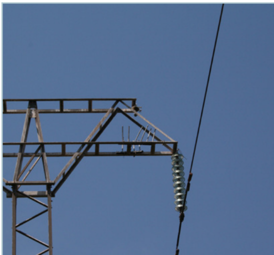
Figure 4: Bird guards were not been installed on the top cross arm to protect the earth peaks. Also note that the bird guards have not been installed at the end of the structure to protect the insulator string. Photo credit: The EWT
