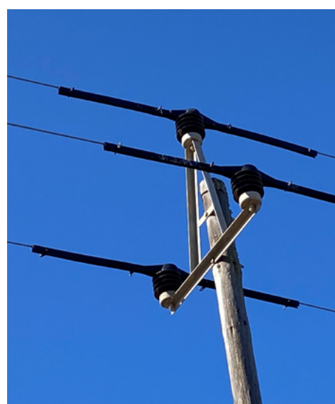
Raptor protectors fitted to a steel A-frame structure. Photo credit: Lourens Leeuwner
