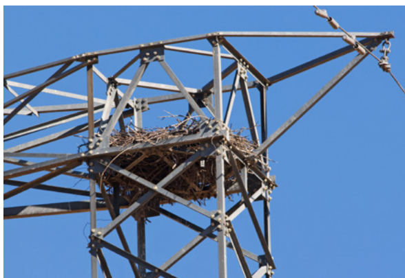
Eagle nest on a transmission tower column. Photo credit: Ronelle Visagie
