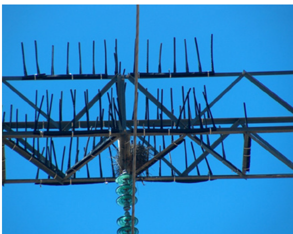
Kestrel nest located above center phase in between bird guards. It is important to ensure that products are fitted correctly and that routine maintenance is carried out. Photo credit: Constant Hoogstad
