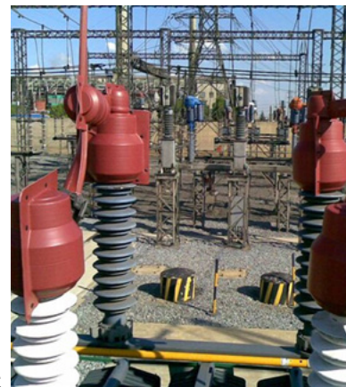
Insulation of the bushings inside a substation. Photo credit: The EWT
