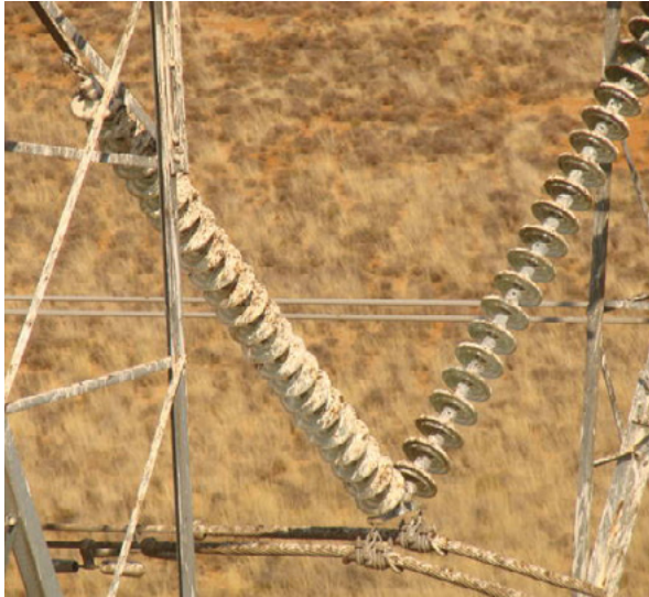
Build up of pollution (bird feces) on insulator strings. Photo credit: Eskom
